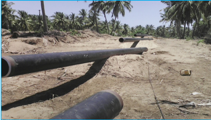
Picture 19: Traditional coconut trees cleared to pave way for gas pipelines from Mtwara in November 2014.
