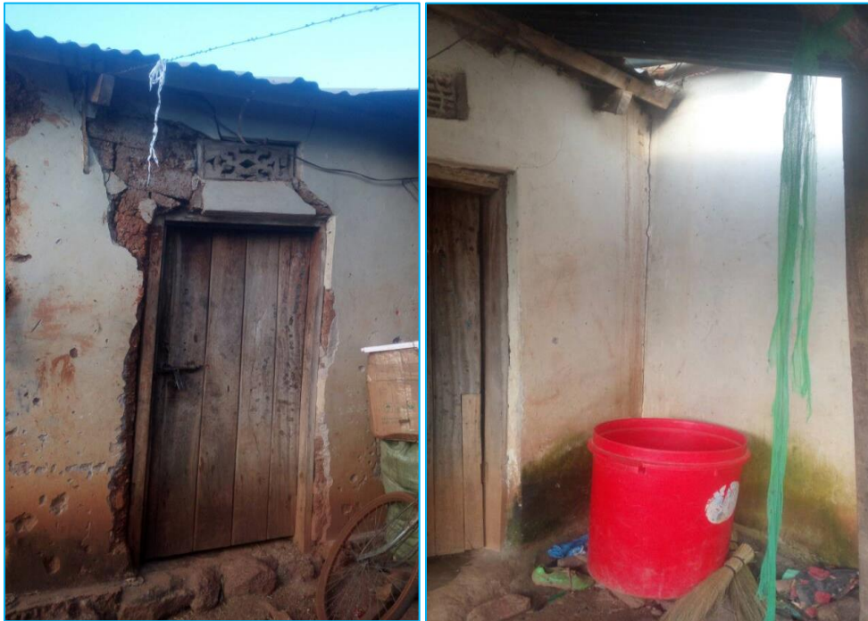
Picture 19: Cracks at some of the houses in Nyarugusu area claimed to have been caused by Pamoja Gold Mine operations
