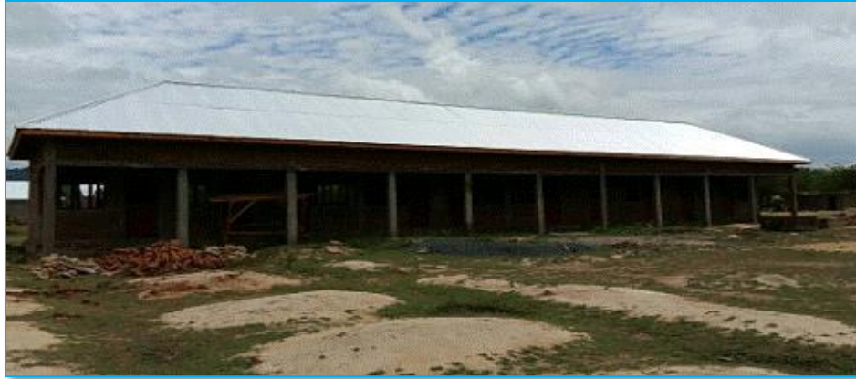
Picture 27: Masware Dispensary, which is under construction, sponsored by Manyara Sugar Company
